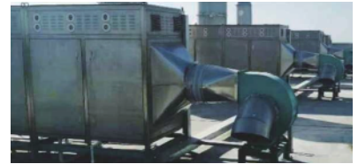
微波光氧除臭设备 Pulse Dust Removal System
